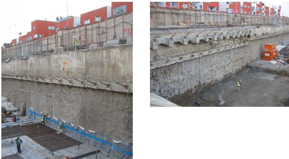
Figure 6. Construction at Smithfield (a) Typical approach and (b) near Queen St watermain
