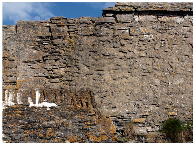
Figure 4. Remnants of vertical coping on face of west pier (Shotton, 2016)
