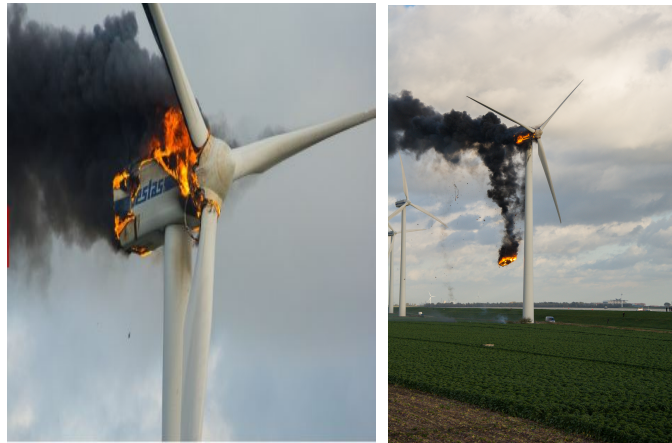
Fig.2 Fire in Wind Turbine
