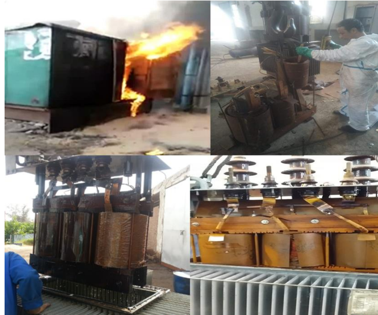
Figure 3. Some symptoms that indicate the deficiency of insulation system inside DTs.
