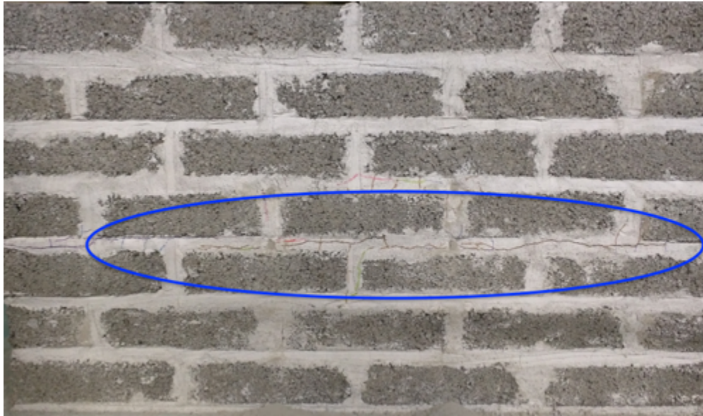
a) Crack propagation photo
