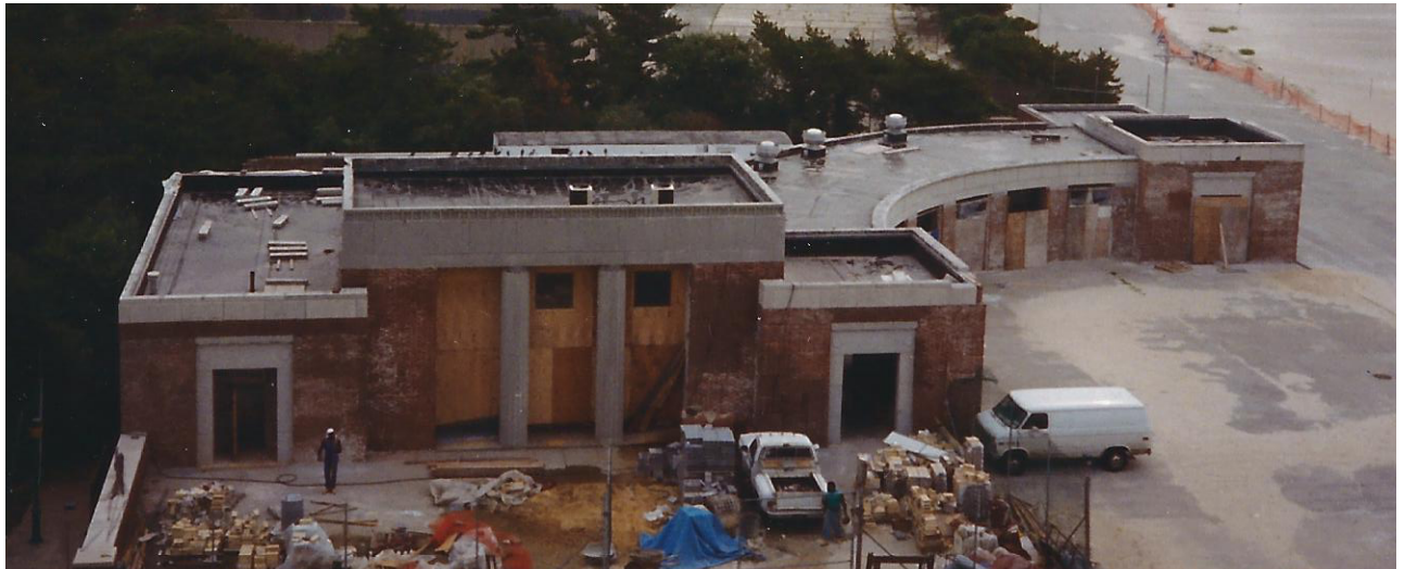
Fig. 1. Half of Jacob Riis Bathhouse Used as a Source for Masonry Unit Reclamation for a Full Restoration of the Mirrored, Counterpart Structure further up the Beach.
