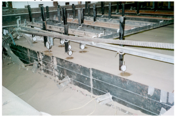
Fig. 7. Top layer of disengaged anchor plates shown during the excavation. Excavation levels shown on the excavation wall as white lines.
