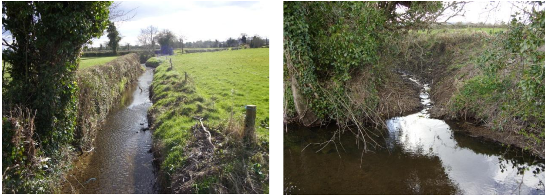
Figure 4 An example of land drains entering a water course on a farm near Mountmellick, County Laois
