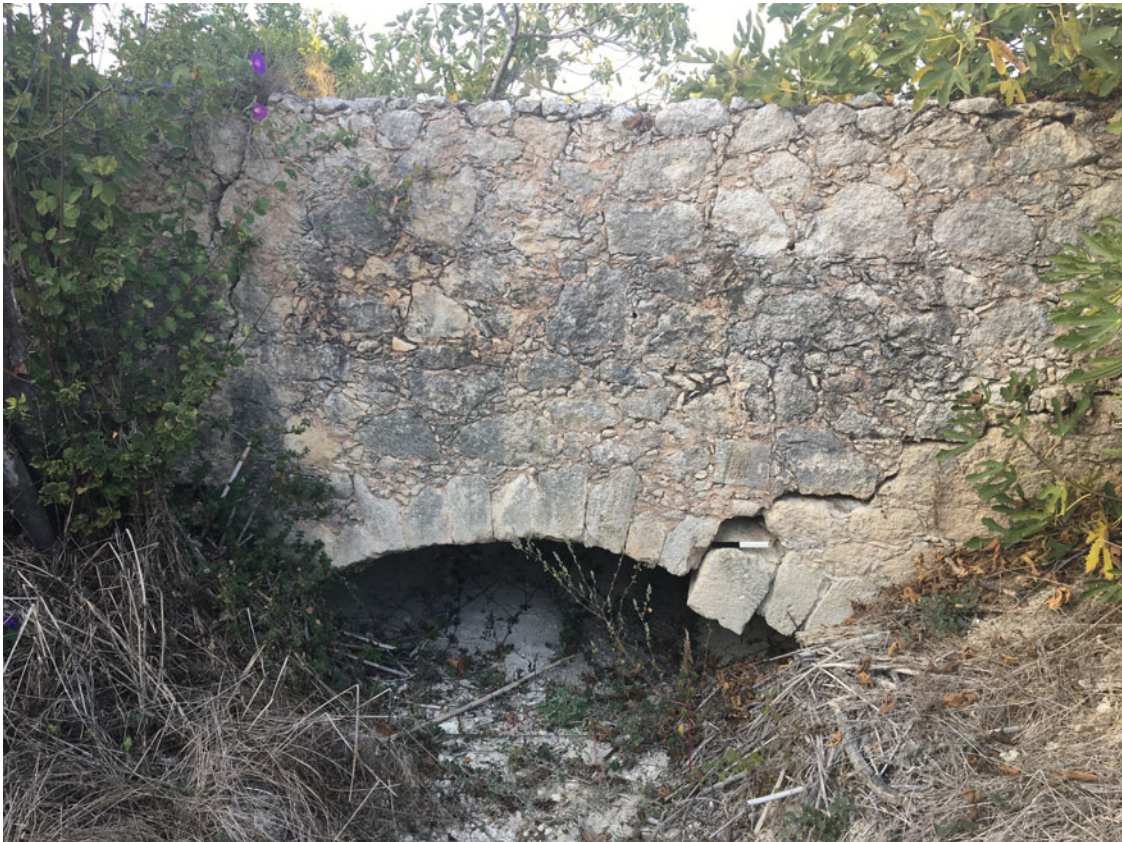
Fig. 12. Ampela Bridge 1, south face. Note crack and slipped voussoirs along right side.
