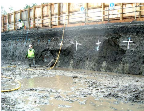
Figure 13. Blocky and highly fissured Dublin Boulder Clay found in the top 3m at Chainage 1250E to Chainage 1265E. This led to local overbreak in cut slope
