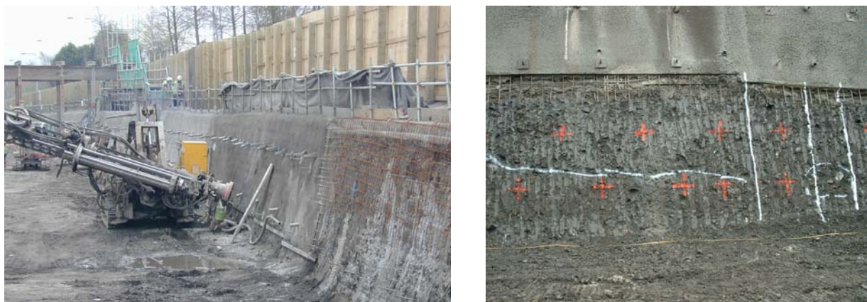
Figure 12. Soil nailed slope under construction at Chainage 1300E, (a) Lift 1 and (b) Lift 2
