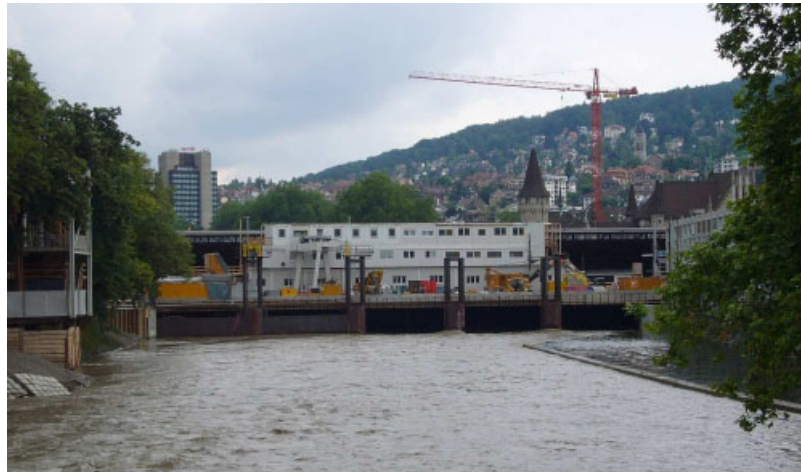
Figure 1. The river Sihl flowing below the central railway station of Zürich. Two of the five channels are closed by tide gates to allow the construction of new track below the river. Picture by A. Badoux, VWSL.
