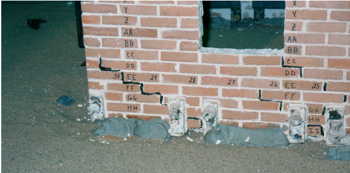
Fig. 15. Close up of damaged URM wall at end of testing; cracks coloured post-test with marker after being measured.
