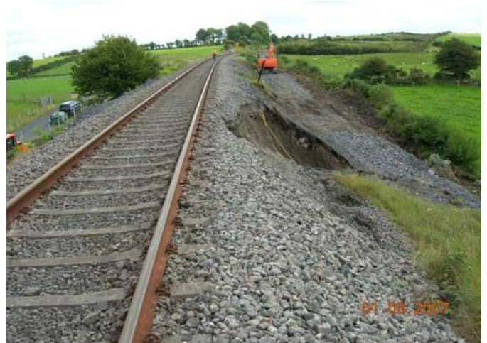
Figure 7: Slope failure near Castlebar, Co. Mayo
