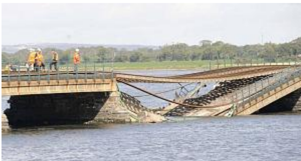
Figure 2: Collapse of Malahide viaduct
