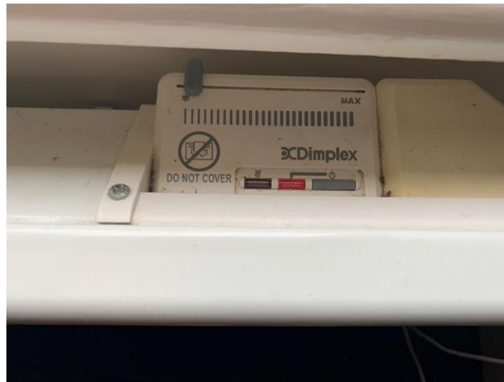
Figure 1. Heater in the Belgrove residence
